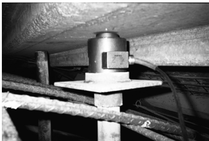
FIGURE 4 Load cell reading in progress
